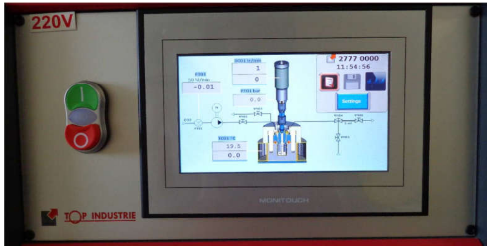
12 13 14 15 16 17 18 19 20 21 22 23 24 25 26 27 28 29 30 31 32 Figure 2. Control cabinet. Source: Authors 33 34 35 36 37 38 39 40 41 42 43 44 45 46 47 48 49 50 51 52 53 54 55 56 57 58 59 60
